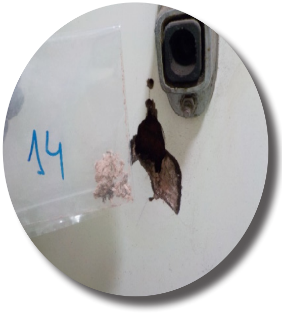
Figure 6: detail of accommodation panel with asbestos fibres (chrysotile)
