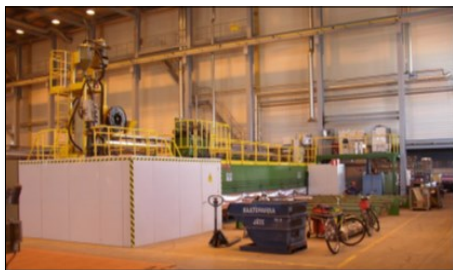
Figure 3. Cell upgraded at AKER YARDS Turku in 2006 for butt jointing through plate butt welding technology in the panel line.
