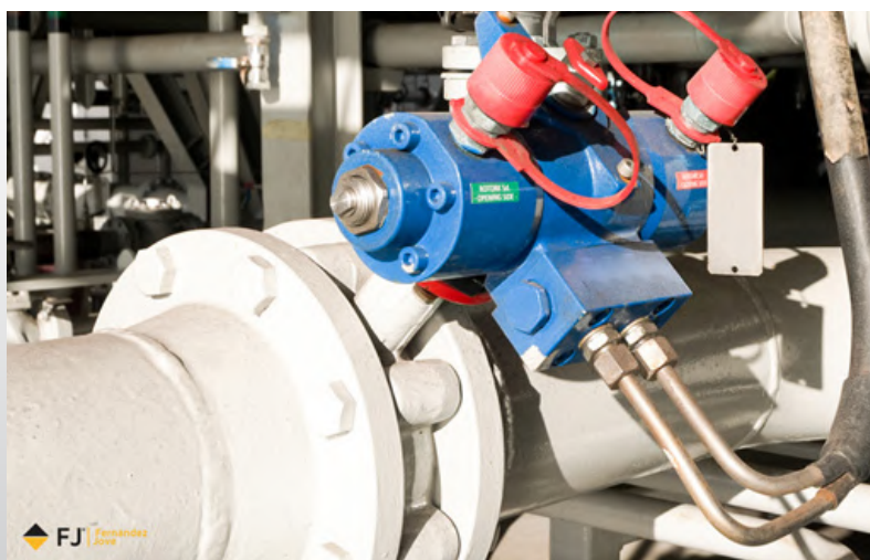
Figure 4. Hydraulic actuator on butterfly valve
