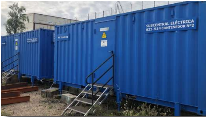
Figure 3. Provisional portable substations used for the bypass of the main building.
