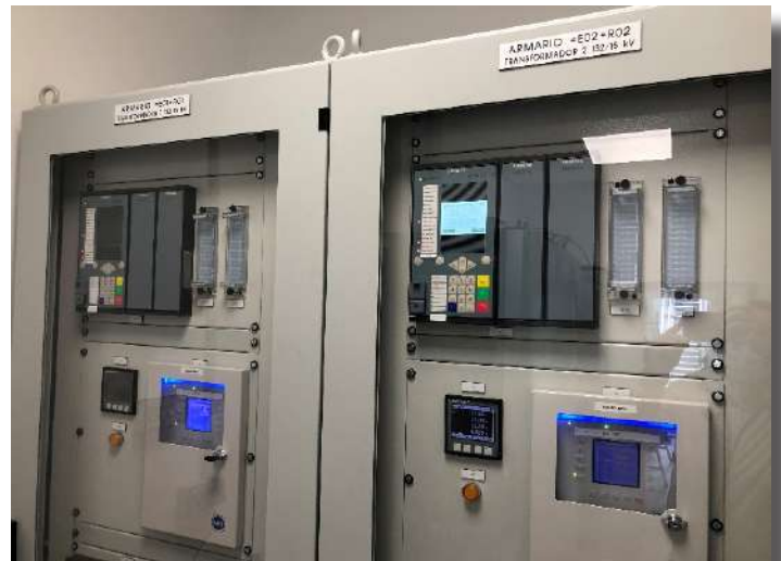
Figure 14. Detail of 132 kV positions.
