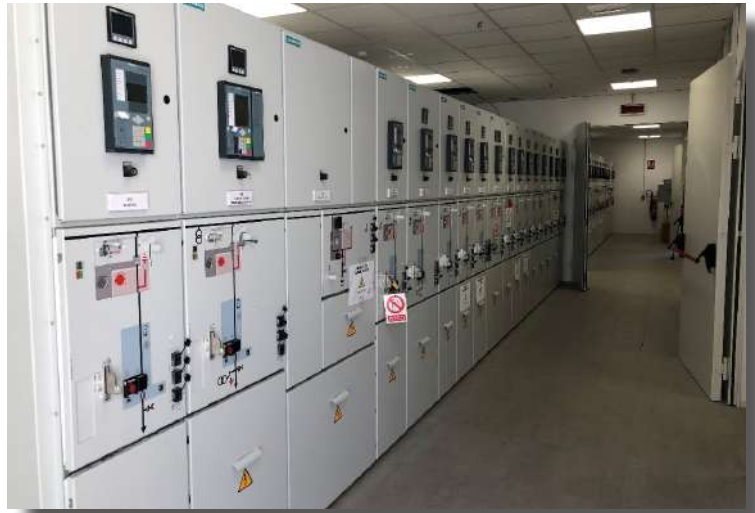
Figure 7. General view of the new operation and control rooms.
