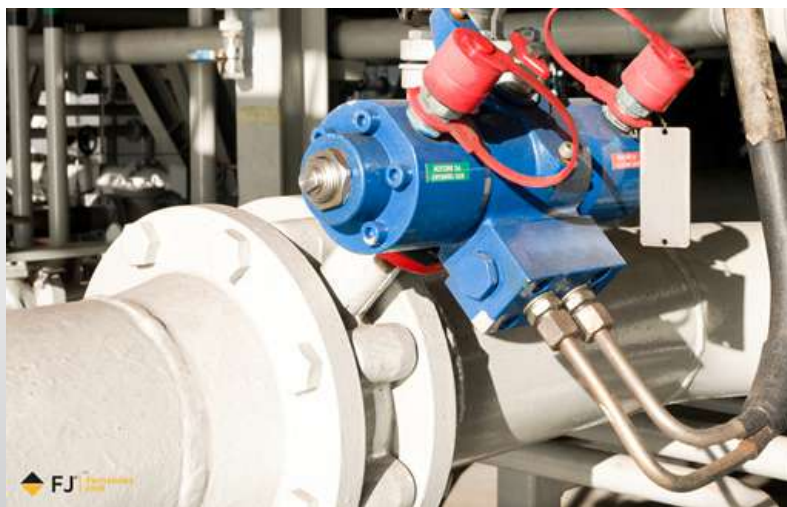
Figure 4. Hydraulic actuator on butterfly valve
